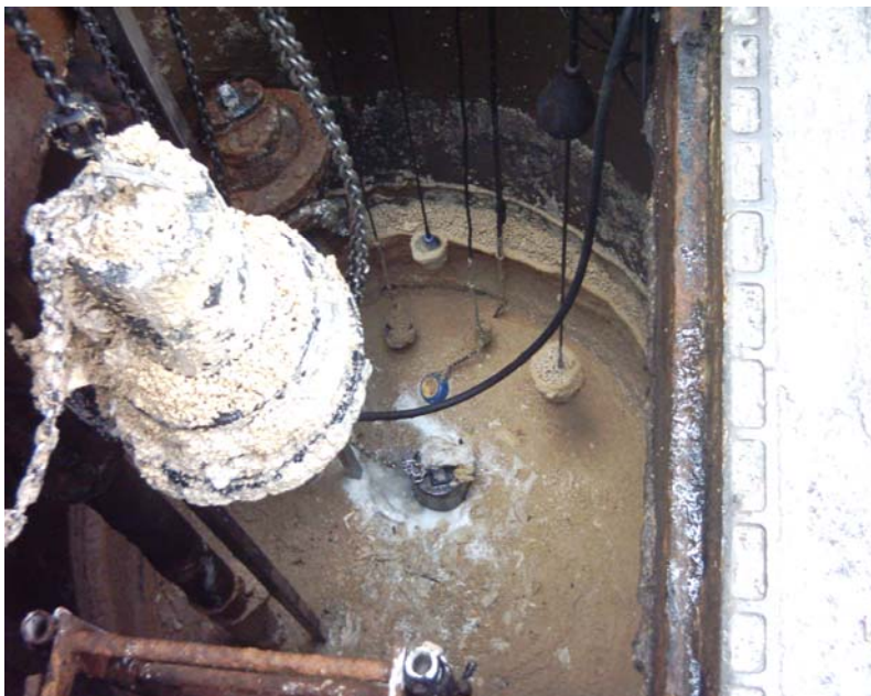
Pumping station blocked due to discharge of oil and grease
