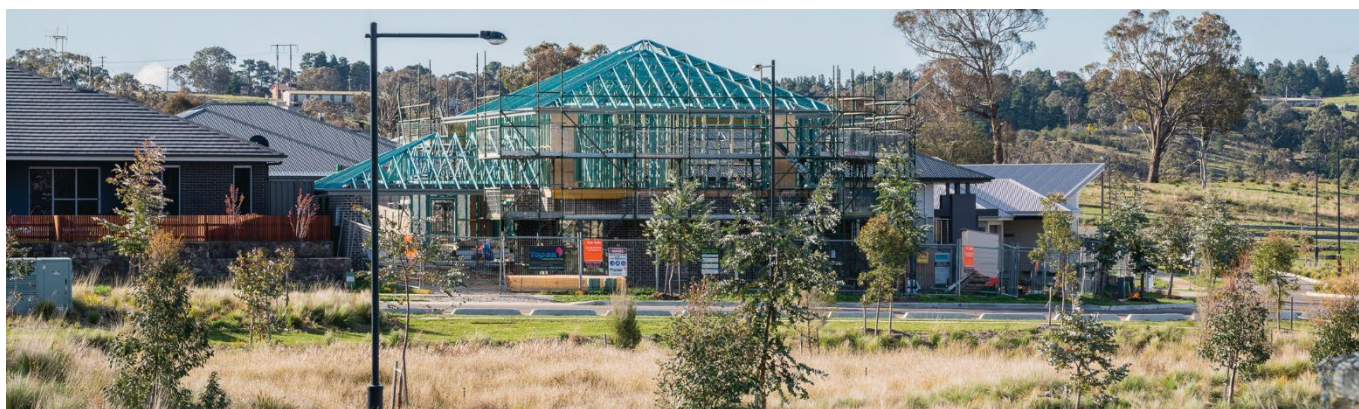
New housing under construction at Googong. Image credit - Jaime Plaza van Roon/DPHI
