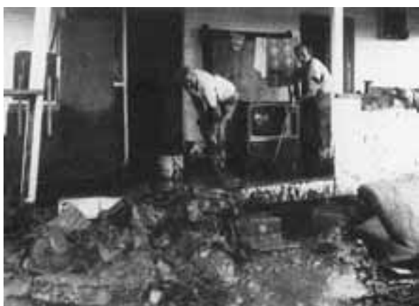
PLATE 5 – Lismore 1974 (Clean up of debris)
